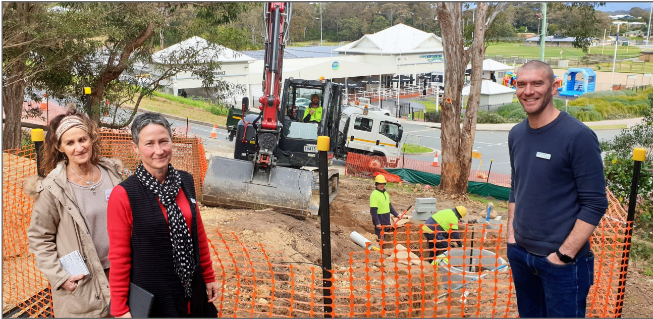
Narooma School of Arts President Jenni Bourke, Eurobodalla Deputy Mayor Alison Worthington and Mayor Mat Hatcher check out the sewerage work underway over the past few weeks to service the new NACC building. The Council crew was Harry Dixon (plant operator), left, Brett Vaughan and Tyrone Thomas. Also on site was Construction Supervisor Lloyd Clarke.
